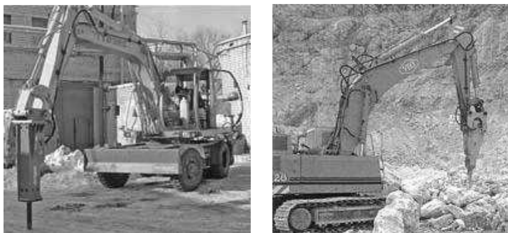
Figure 1.8. Hydraulic hammers V in the process works
