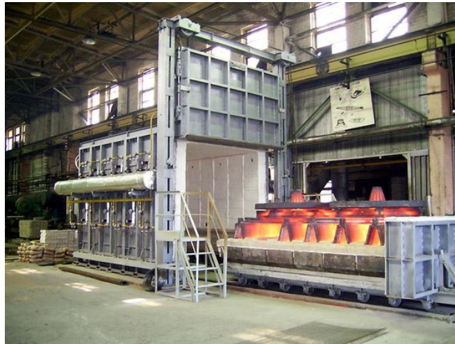
Figure 16.5 – Chamber gas furnaces for heat treatment
