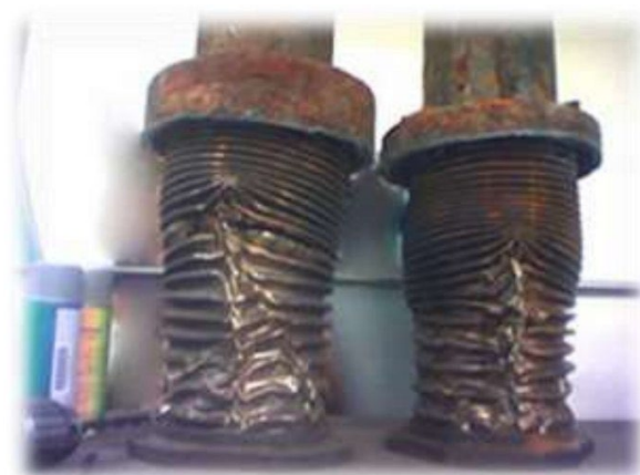
Figure 3. Deformation of pipeline transition branch pipes caused by water hammer
