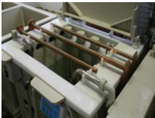
Fig. 8. Installation for galvanic chrome plating
